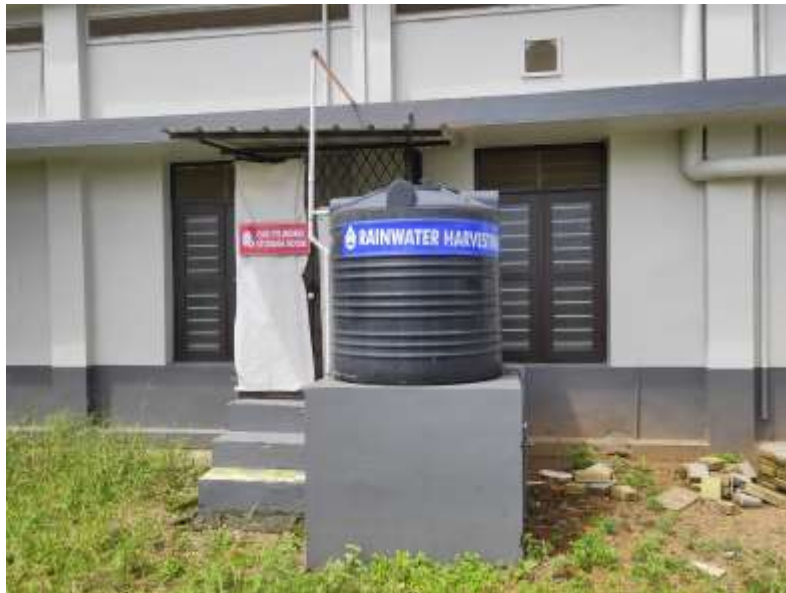
Figure 13 RAIN WATER COLLECETION
