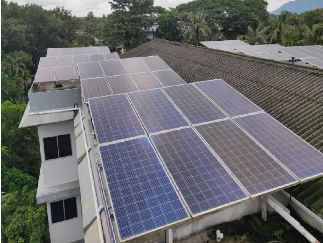
FIGURE 14 : ROOFTOP SOLAR PV SYSTEM
