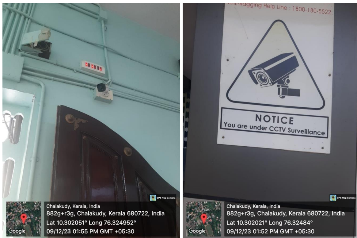
CCTV Cameras installed in each floor
