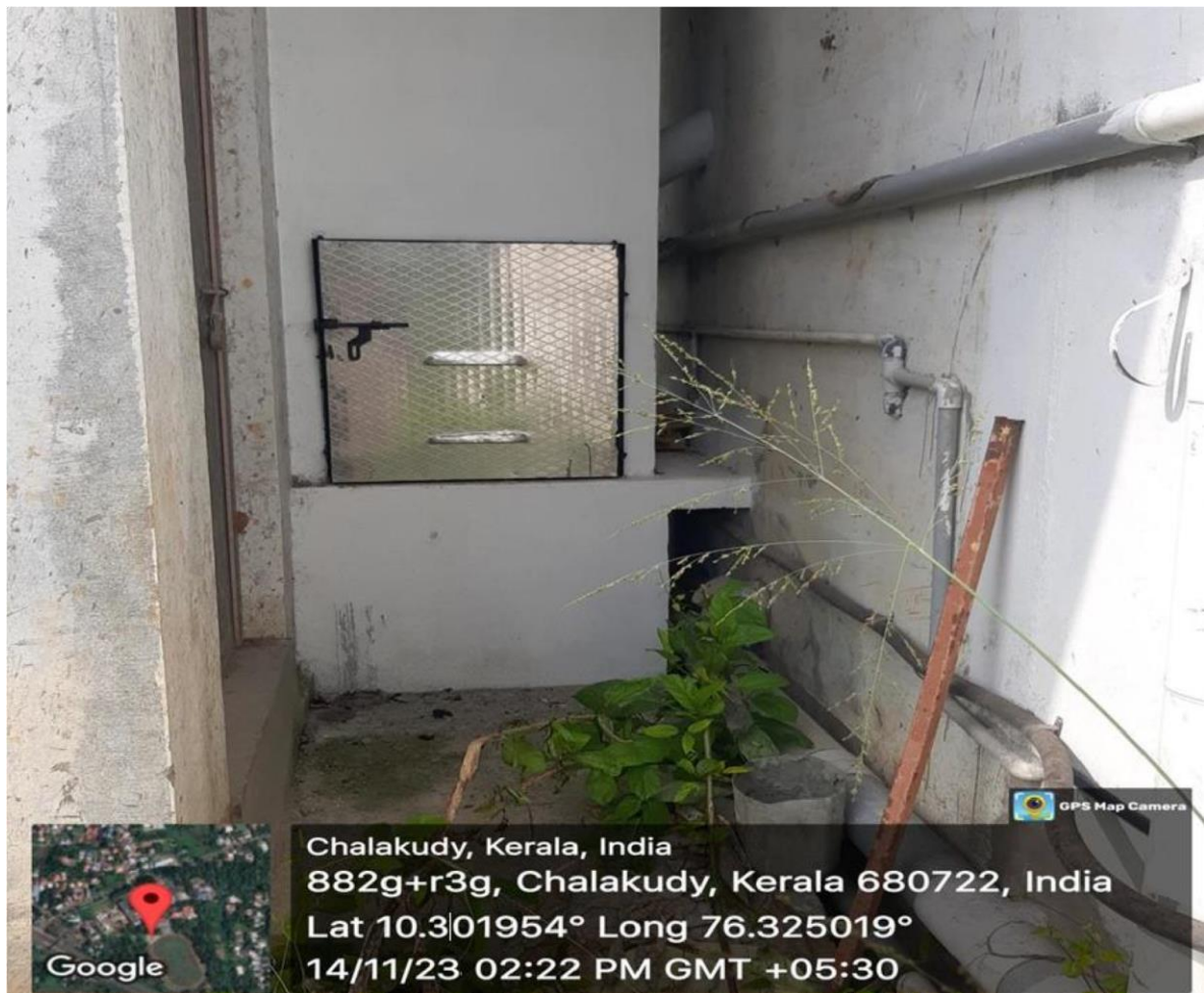
Geotagged photograph of safe disposal of sanitary napkins using incinerator
